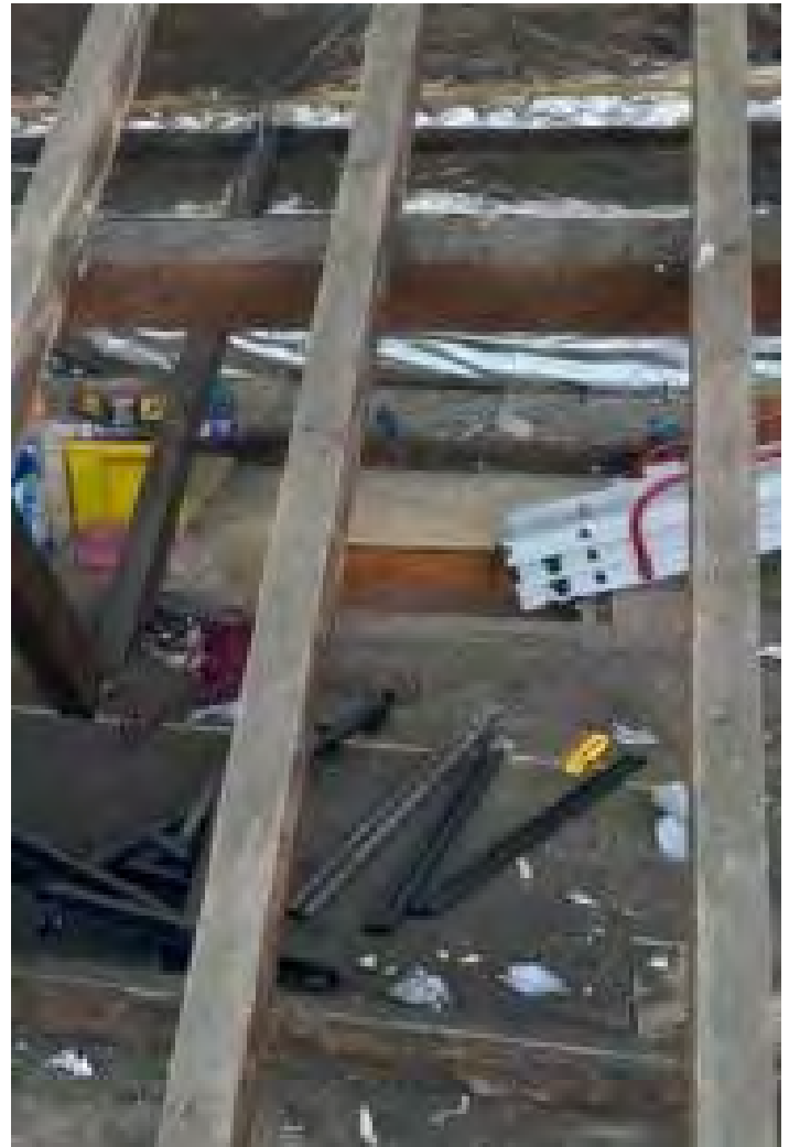
Image: HSE - The unguarded loft hatch
